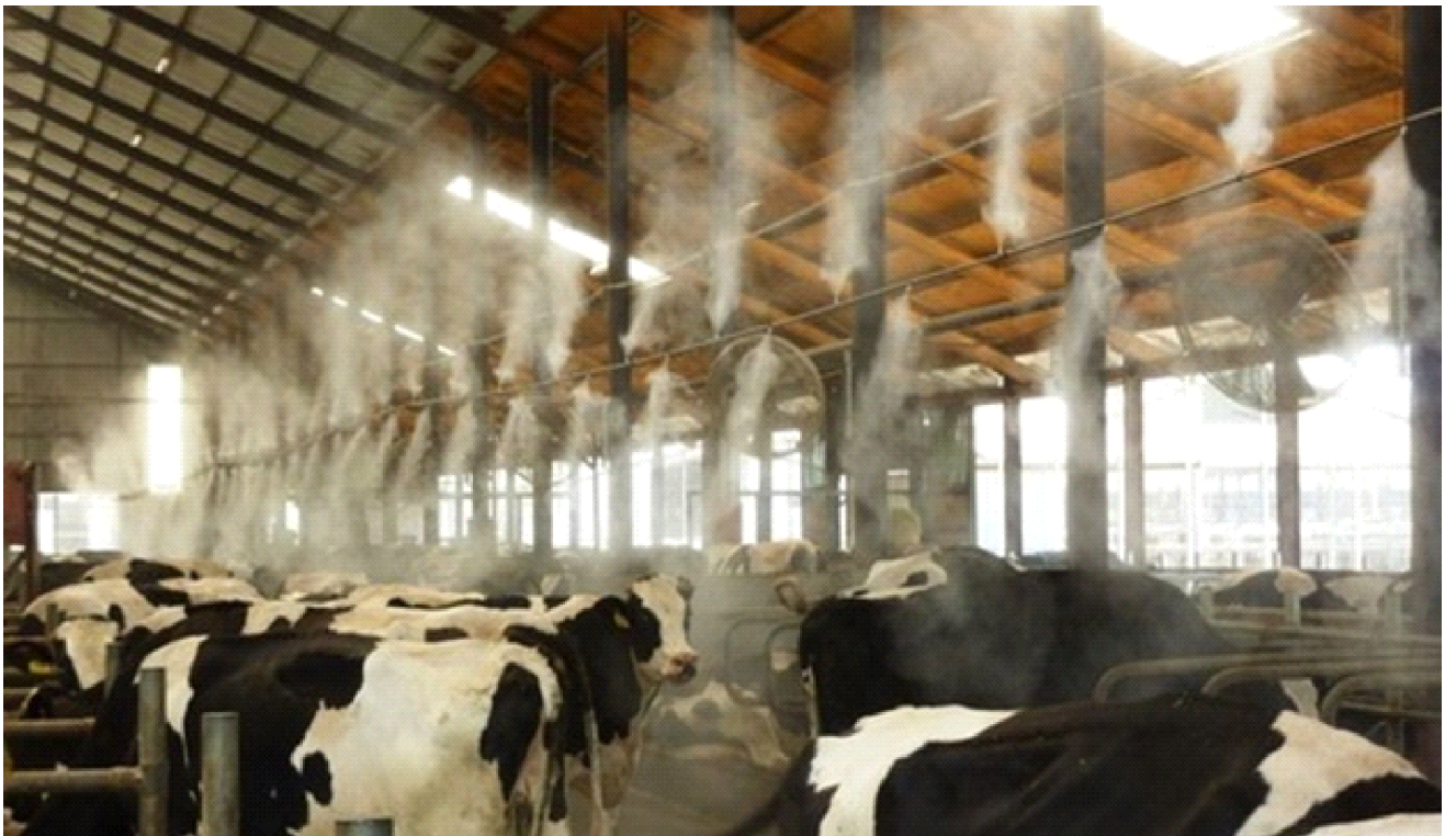
Photo 1. Fogger system in livestock shed
